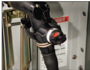
A Test Point Reset Fault Indicator with junction shield provides indication in a switchgear cabinet.
